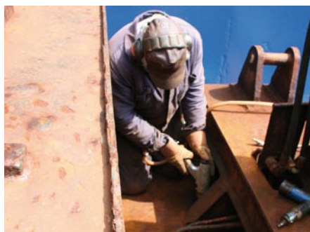
Personnel descaling rust need to take regular breaks to rest their bodies.
