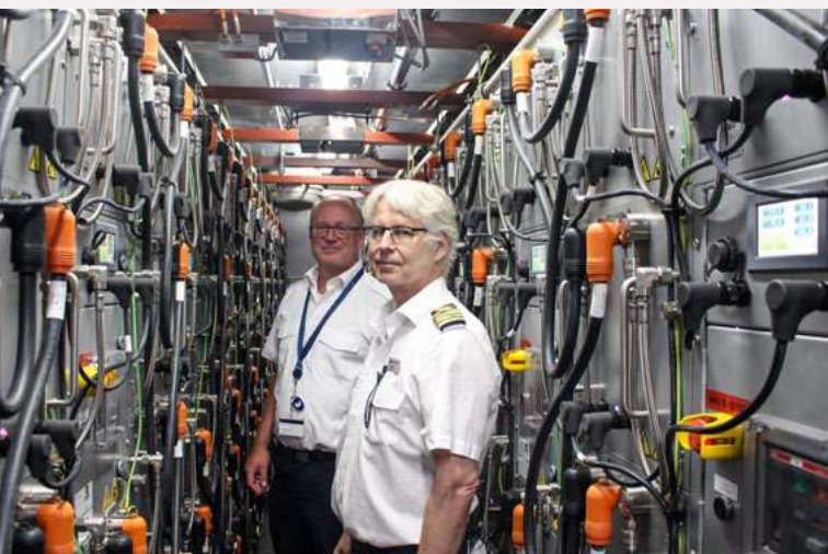
Christian Andersson (left) and Robert Möller inside one of Aurora's four battery containers.
